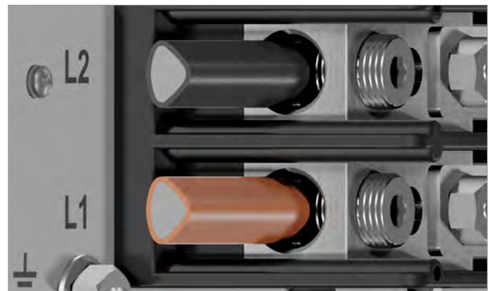
Correct position of sector-shaped aluminum cables (2)
