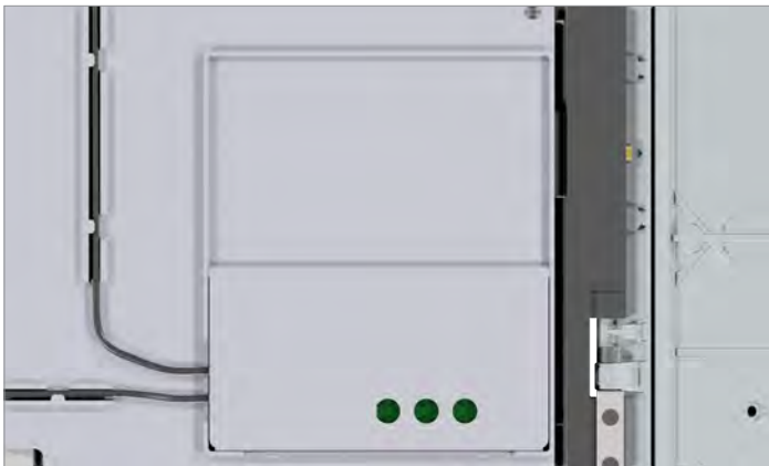
Fig. 4.10: DC surge protection devices
