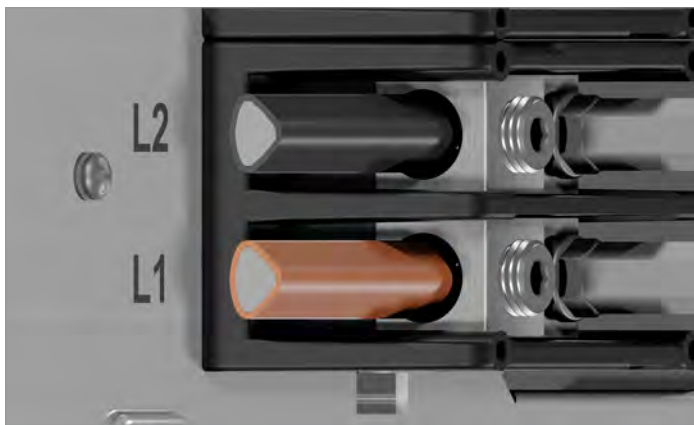
Correct position of sector-shaped aluminum cables (2)
