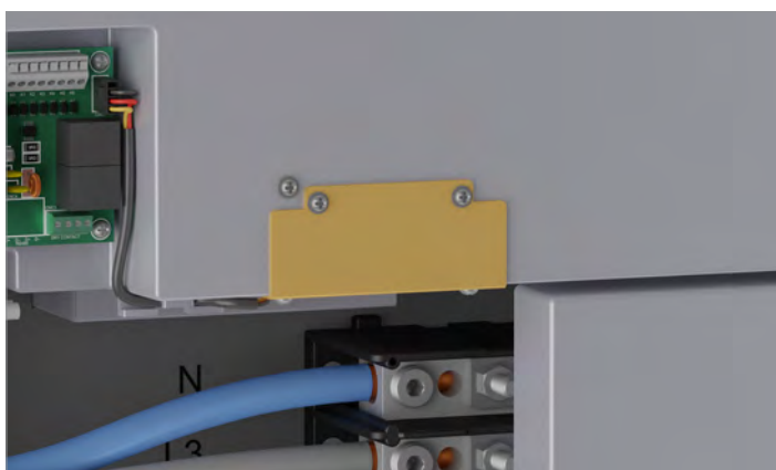
Position of internal fan 1
