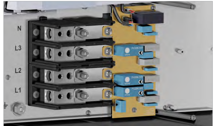
Fig. 4.6: View of type 2 AC surge protection devices with the cover removed
