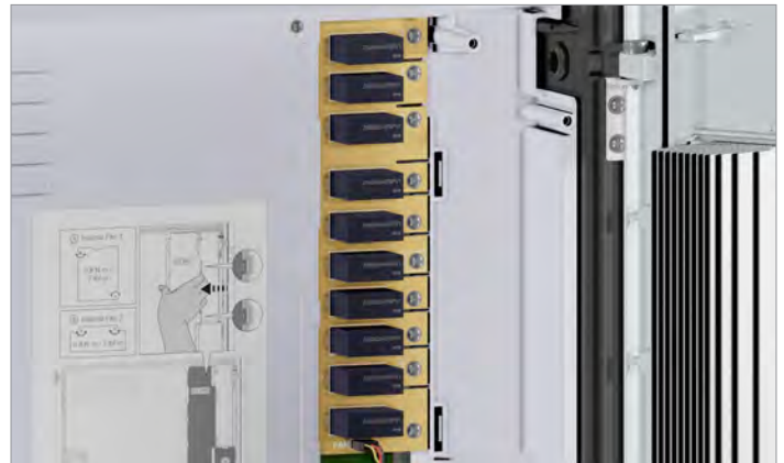
Fig. 4.14: View of the DC surge protection devices with the cover removed
