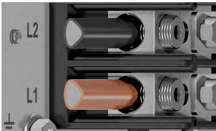
Correct position of sector-shaped aluminum cables (2)
