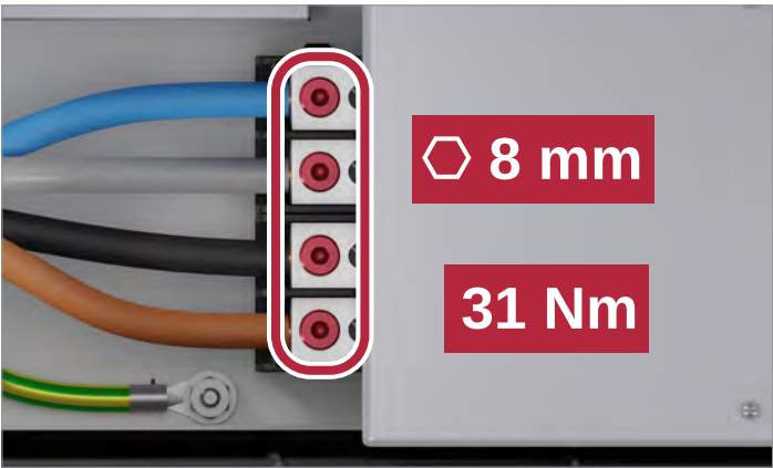
Torques at the AC terminal block
