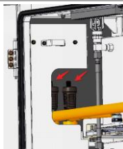
Figure 7.1: Automatic air vent valve cap at the top of the liquid cooling piping outlet
